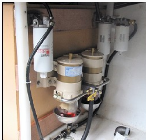
Multi-Stage w/ Racor's and fuel transfer polishing system
