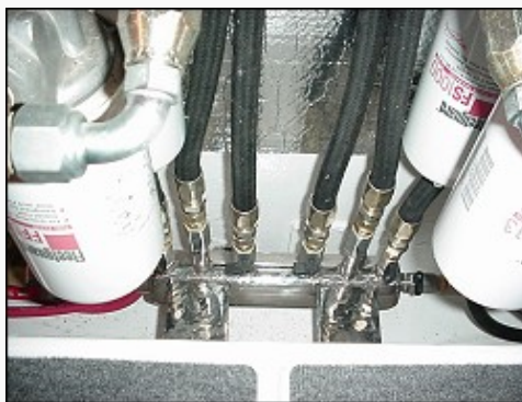
"No Diesel Sweat" - Fuel Manifold w/ 100% epoxied fittings / threads
